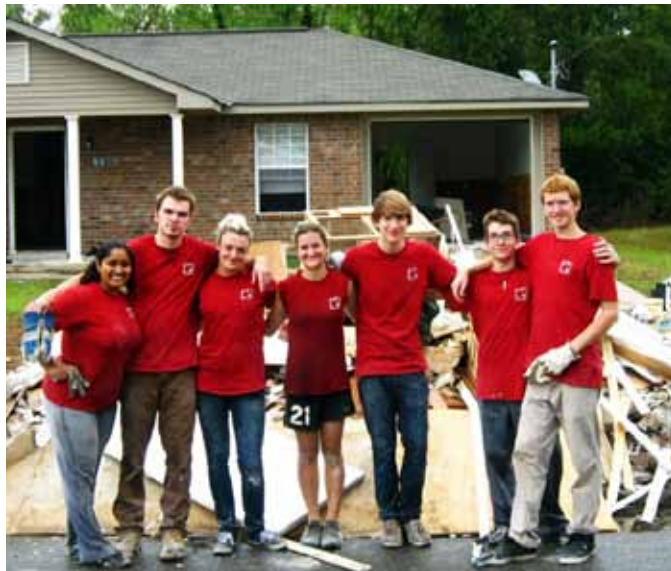
LUCAP students gut a home in LaPlace, Louisiana after Hurricane Isaac (Fall 2012); Credit: Loyola University Community Action Program
