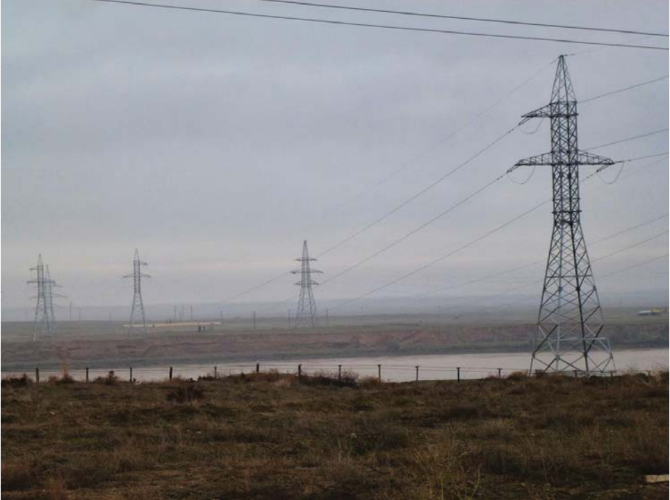
Photo 3: High-voltage lines crossing over Pyanj River from Tajikistan to Afghanistan
